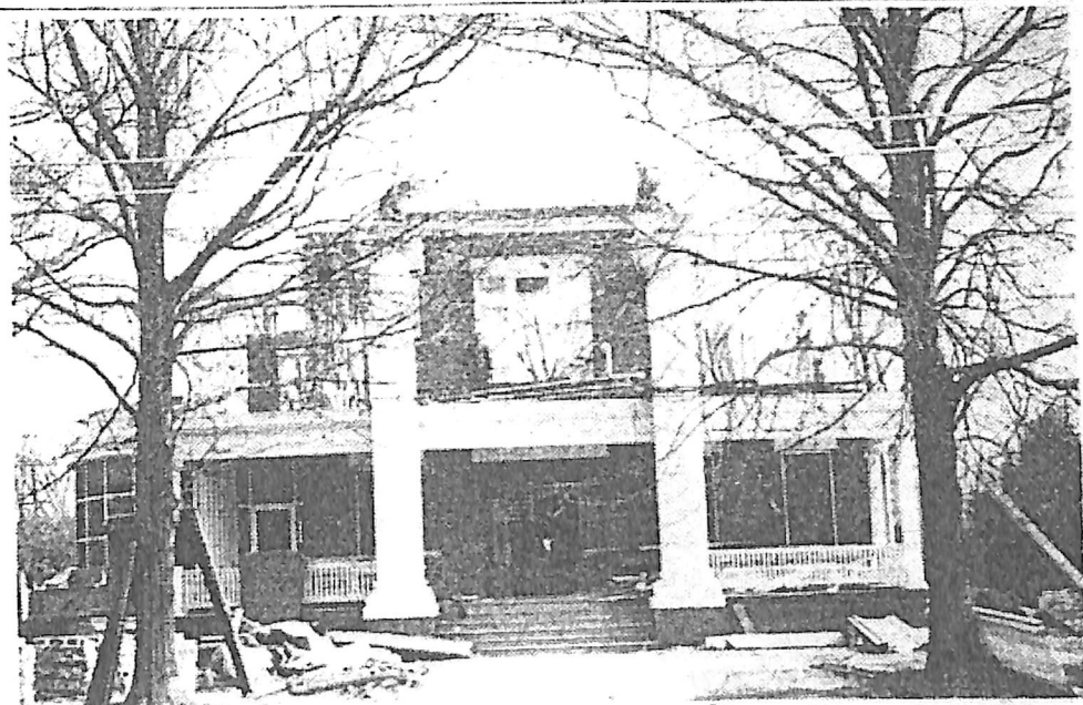
NOW NO MORE —All that was left last week of the former Norman A. Mott home. The 27 foot fluted Corinthian capped columns stand majestically in almost righteous indignation to the demolition that has been in progress since mid-December.
